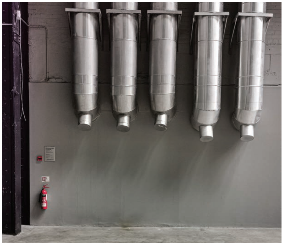
Tate Modern, Fire Extinguisher
